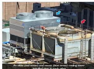
An older (red arrow) and newer (blue arrow) cooling tower installed next to each other.
